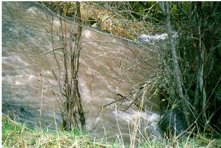
Figure 23. Inadequately sized culvert located in the upper Sweetwater HUC. Note culvert placement/alignment in relation to thalweg.
