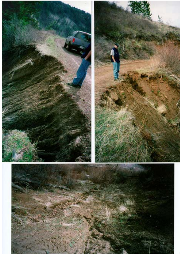
Figure 20. Road slump on native-surfaced secondary forest roads in the upper Sweetwater HUC. Top photos show initiation point, lower photo shows deposition. Surveyed March 2000.
