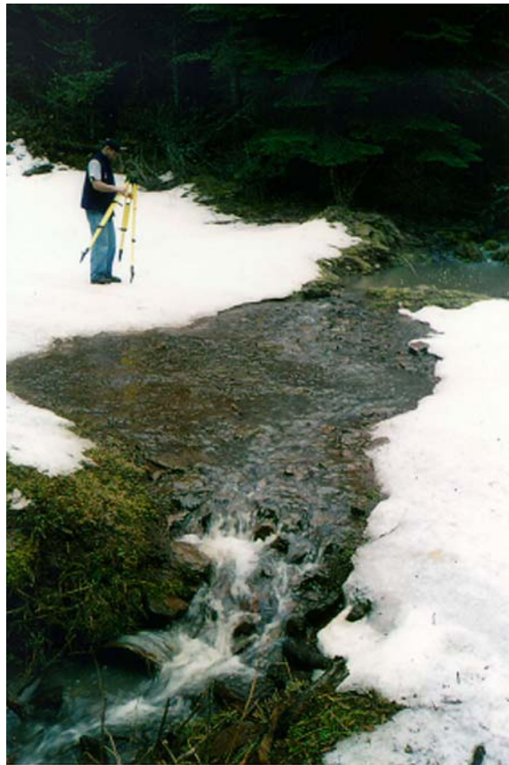
Figure 25. Culvert draining unnamed tributary to the East Fork Sweetwater Creek. Photo illustrates the effect of a crushed culvert inlet and corresponding surface erosion.
