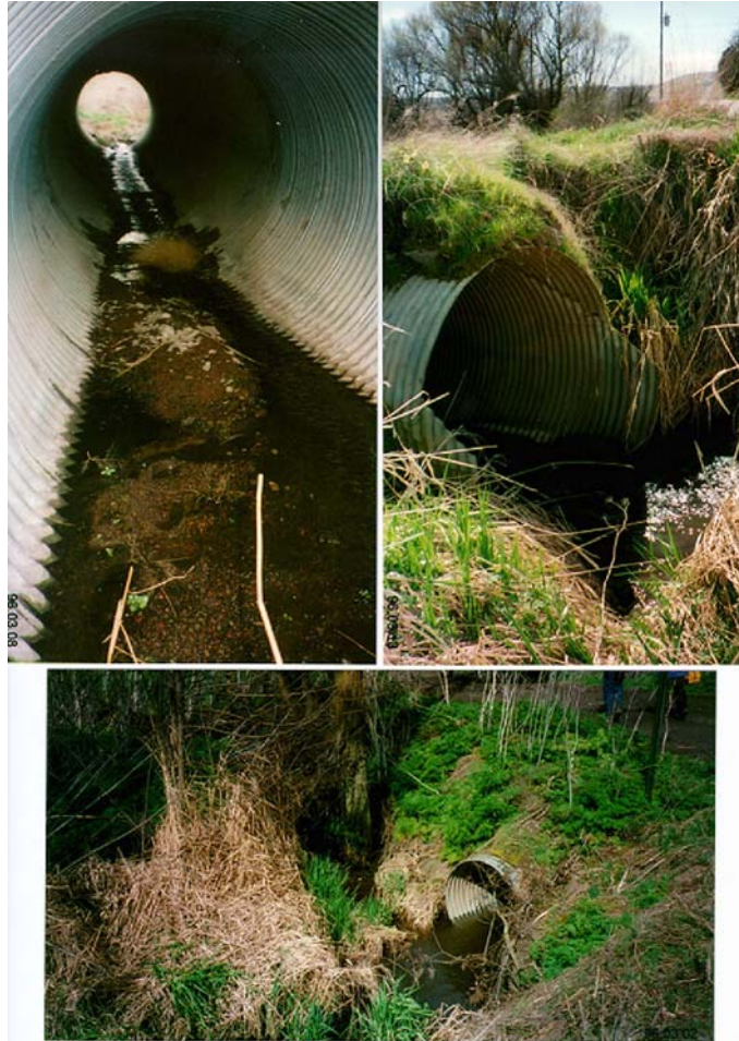
Figure 22. Culverts draining agricultural ground. Culvert locations are (clockwise) Middle Sweetwater, Tom Beall, and Tom Beall. Surveys conducted March 2000.
