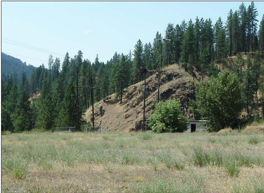
Figure 1, Transformer sites; cinder block transformer building and fenced power poles in background.
