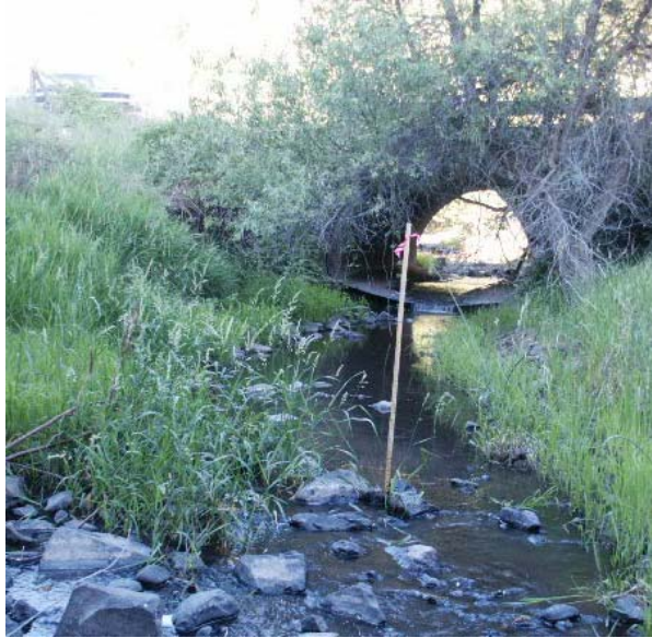
Figure 28. Fish Passage Barrier on Sweetwater Creek in the Lapwai Creek Basin Culvert was recently replaced with bridge.
